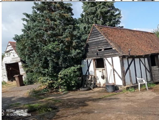
Photograph 3: South-eastern elevations of B2 (left) and B3 (right) in the north-east of the site (Moderate bat potential).
