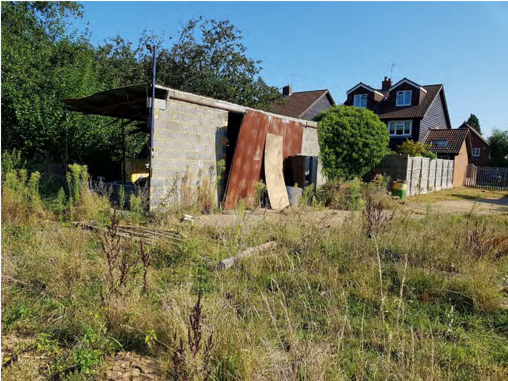
Plate 3: The northwest corner of the building is damaged and part of the roofing is has been removed.
