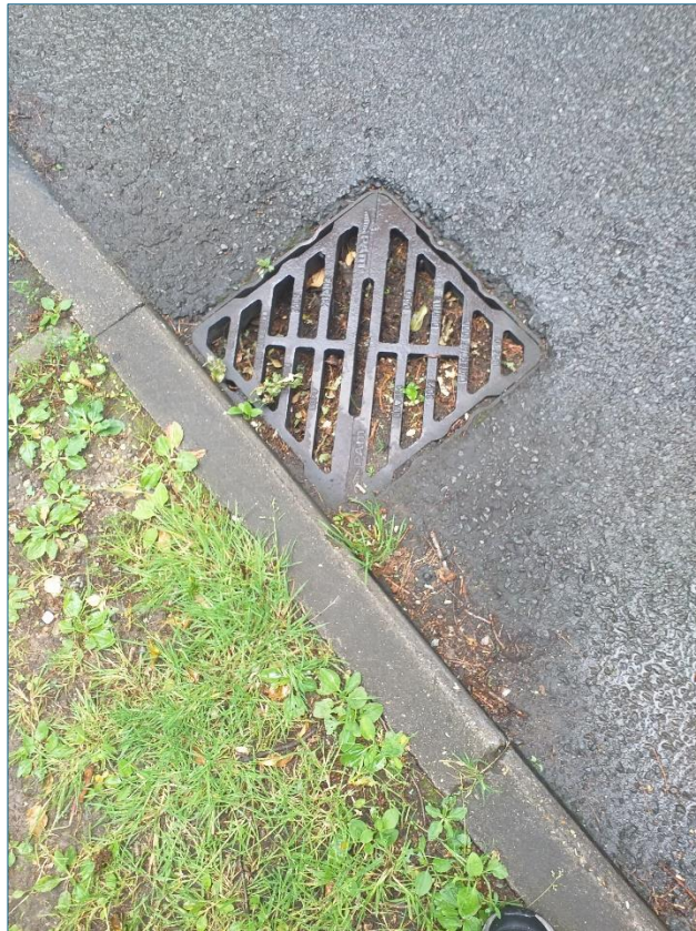
Photo 5 – Blocked storm drain on Park Street Lane
