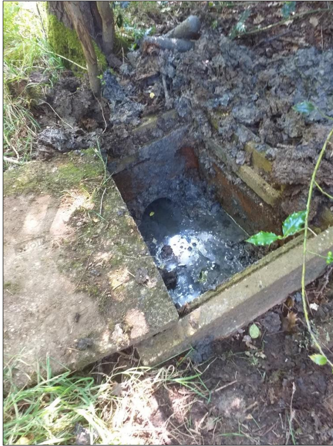
Photo 3: after the catchpit was cleared of mud, the presence of pipes was confirmed and the chamber began to fill with water.
