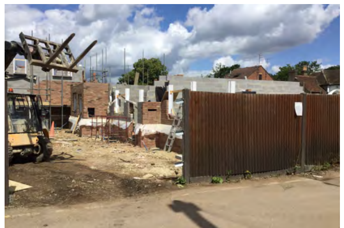
Looking north from southern boundary of sub-area with views of ongoing construction within sub-area
