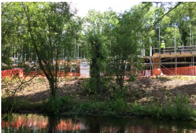
Looking east from Moor Mill Fishery with views across the River Ver towards ongoing construction within the sub-area
