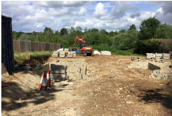
Looking west from east boundary of sub-area with views of ongoing construction within sub-area
