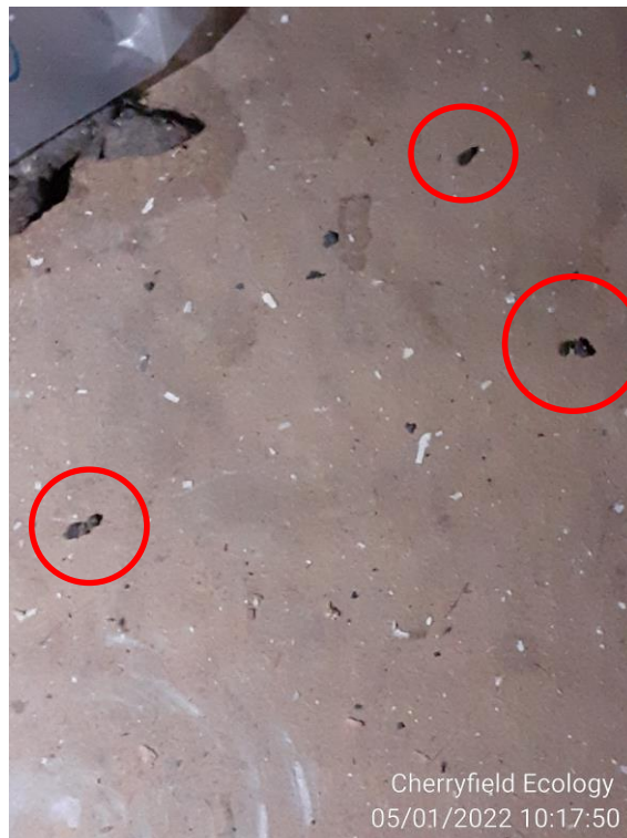
Figure 32: Example of bat droppings in B1
