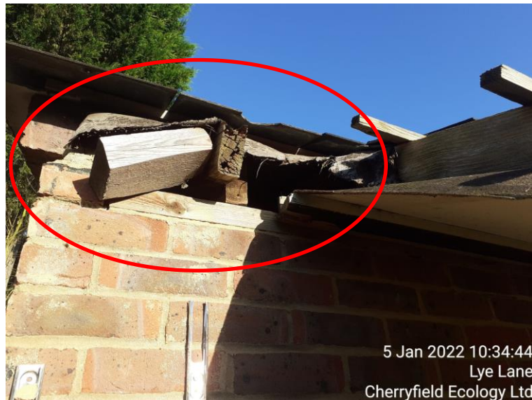
Figure 40: Example of gap at eaves of B2
