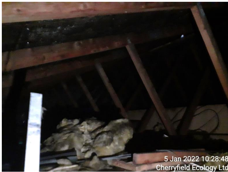
Figure 14: Loft Space 2 of B1
