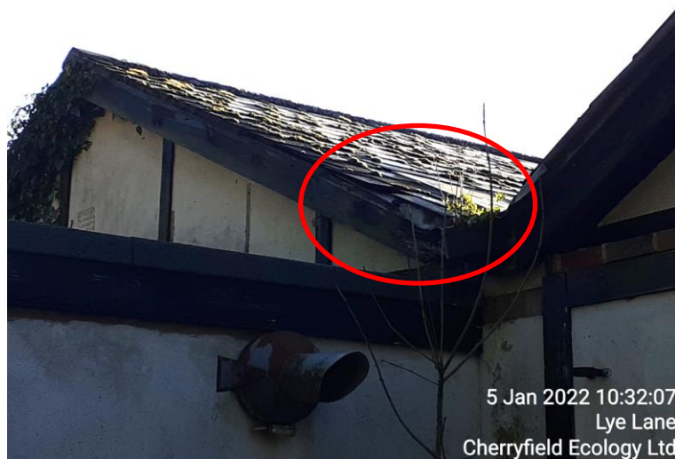
Figure 36: Example of gap between tiles of B1
