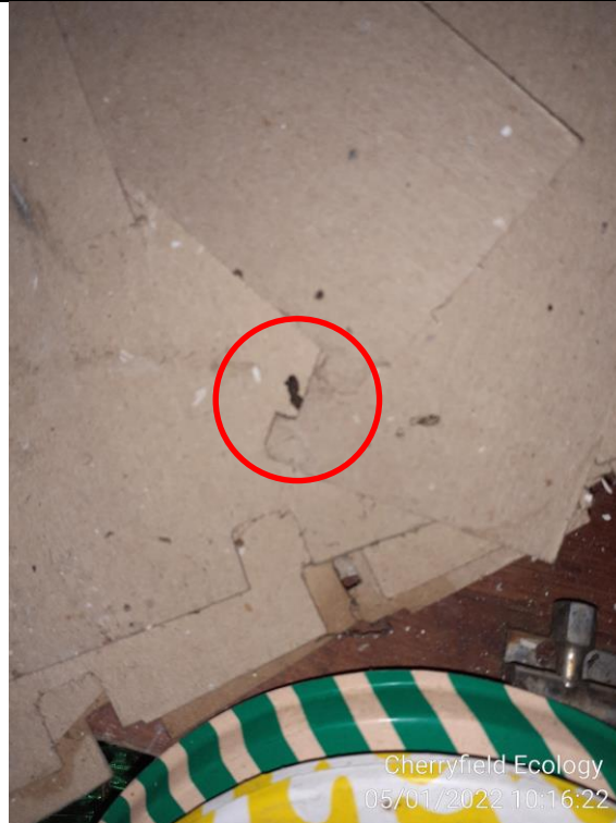
Figure 31: Example of bat droppings in B1
