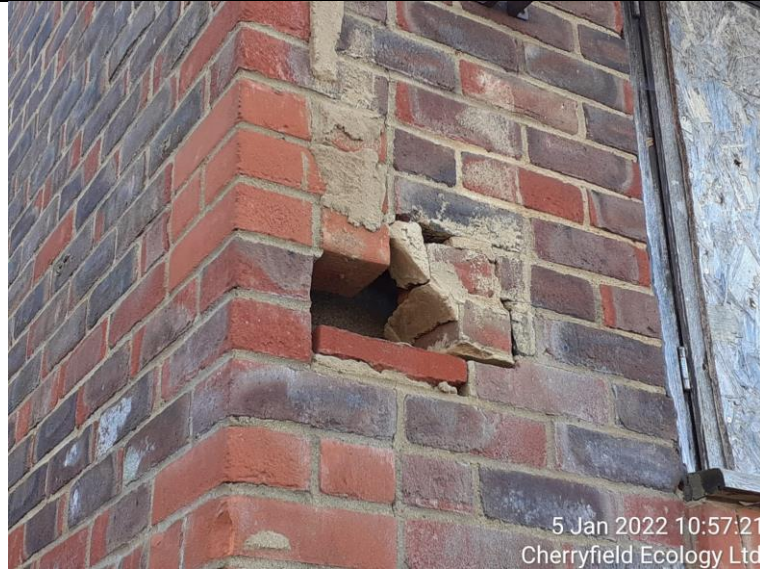
Figure 39: Gap between B3's external brickwork
