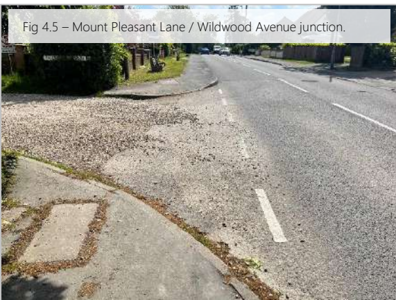
As per Fig 4.3, consider provision of dropped kerbs and tactile paving. Gravel from the private road within the highway boundary, consider increased surface maintenance.
