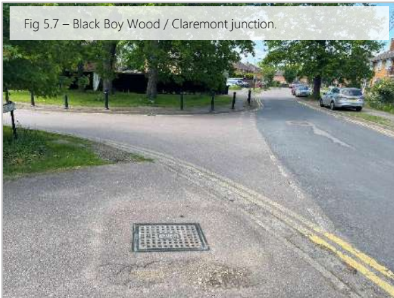
As per Fig 5.1, consider provision of new uncontrolled pedestrian crossing comprising of dropped kerbs and tactile paving.
