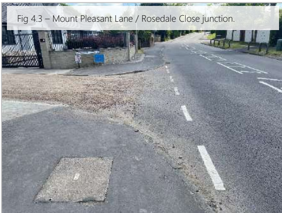
Consider provision of dropped kerbs and tactile paving. Gravel from the private road within the highway boundary, consider increased surface maintenance.
