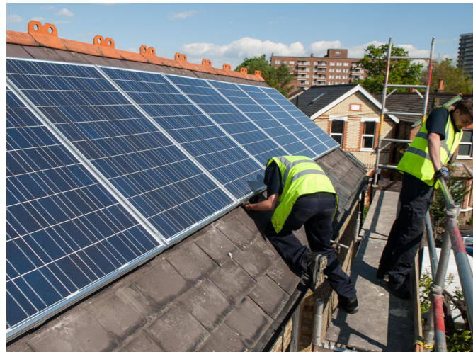
Figure 11 Solar Panel installations
