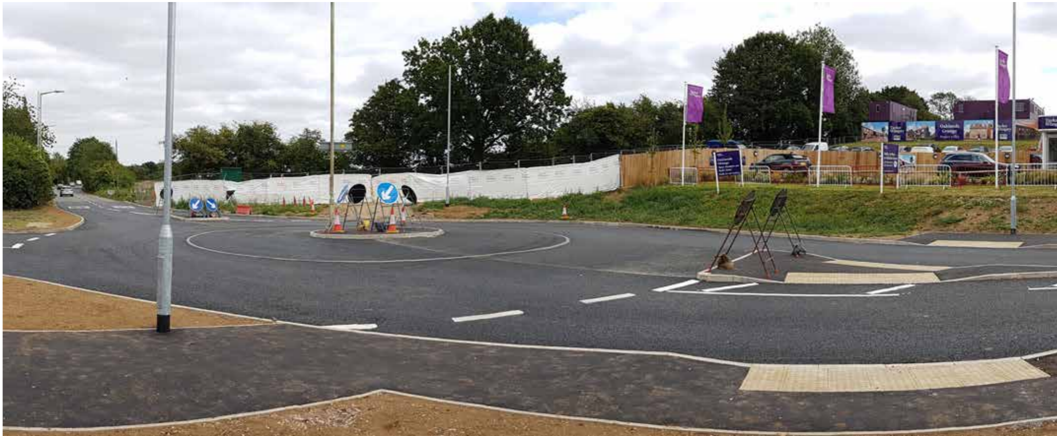
The image above shows the road improvement works to Sandpit Lane, and the entrance area to the new Taylor Wimpey site.
