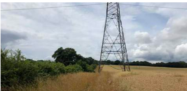
View of pylons
