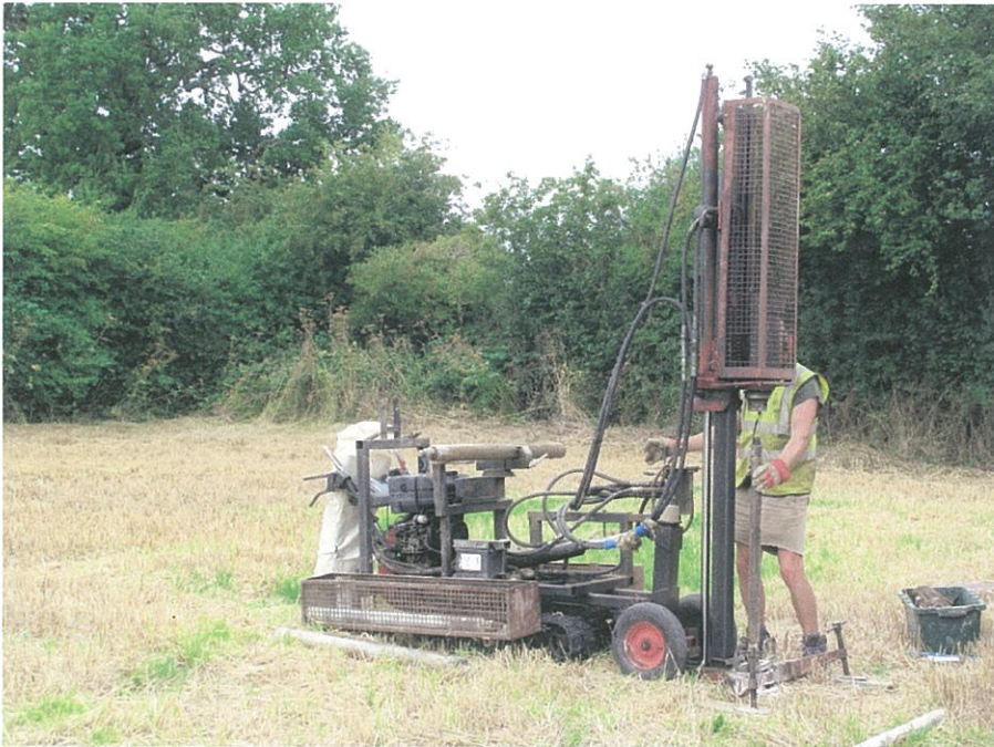
Photo 13: view of WS7 near the western corner of the site during drilling.
