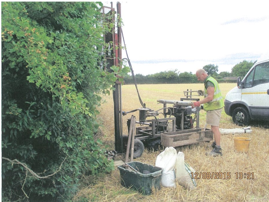
Photo 24: view of WS16 during drilling by the current site entrance, looking north into the site.
