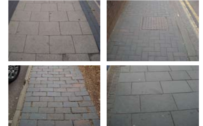
There is a varied palette and pattern for paving materials used in St Albans main streets.
