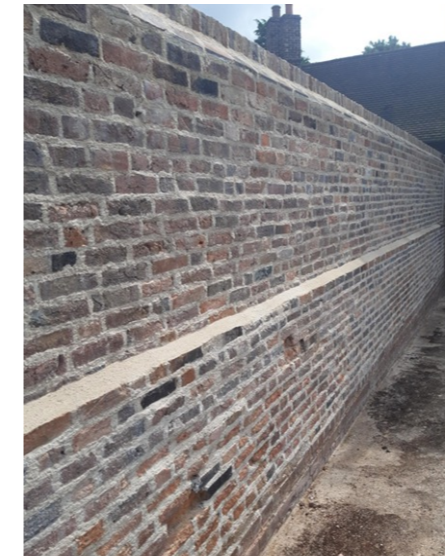
Rebuilt wall to rear of Pemberton Almshouses, St Albans (Grade II Listed Building)
