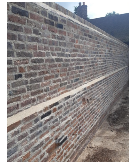
Rebuilt wall to rear of Pemberton Almshouses, St Albans (Grade II Listed Building)
