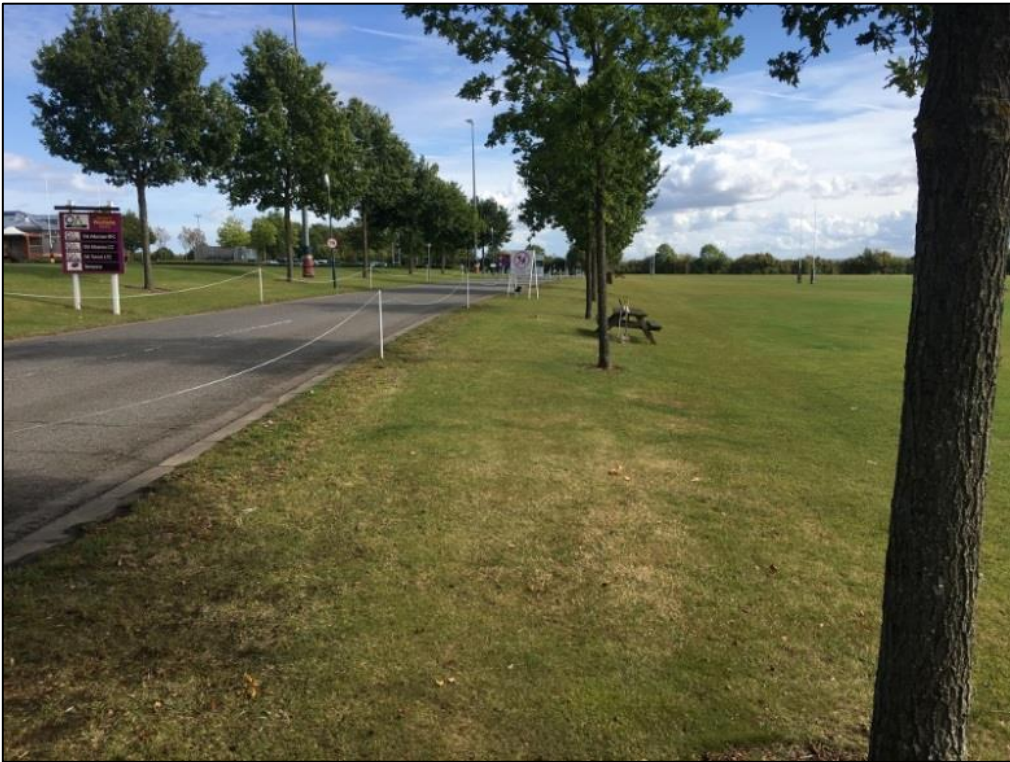
Figure 8 Batter slope down from the access road on to Area A illustrating that cut and fill earthworks have taken place
